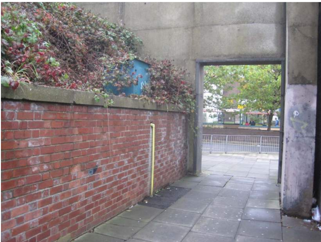
Photograph 4 Yellow pipe protruding from embankment retaining wall. Facing North.
